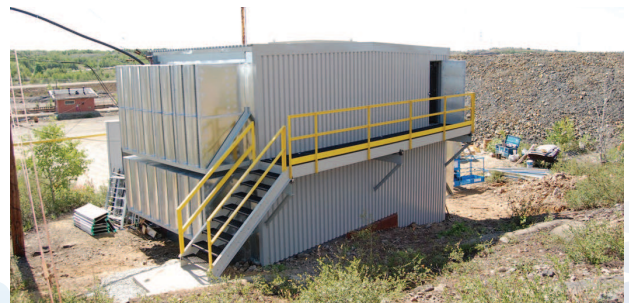
Mine Fan Intake Noise Enclosure
